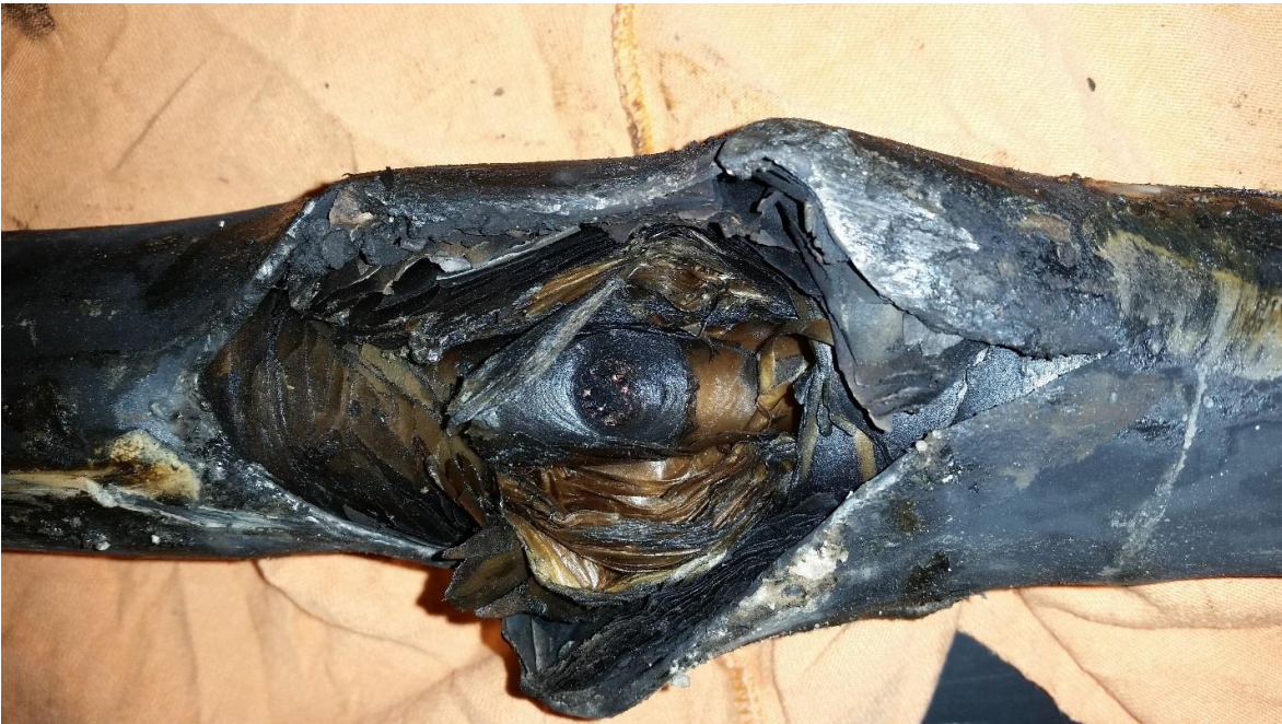
Figure 22, A faulted PILC cable
