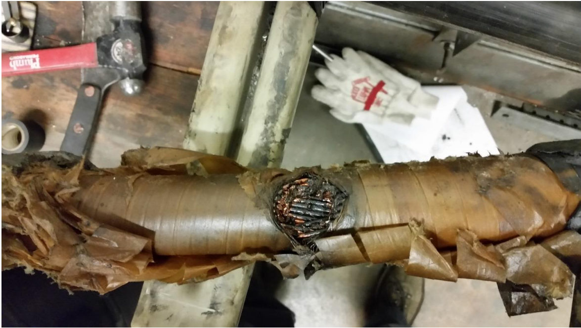
Figure 23, A second faulted PILC cable
