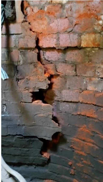
Figure 25, Interior of a badly deteriorated old manhole in a heavily traveled street
